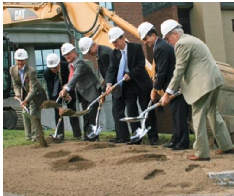
ESF President Cornelius B. Murphy, Jr., right, joins a group of dignitaries as the ceremonial shovels toss the first soil to make way for the ESF Gateway Building. The building will use an array of renewable energy technologies to showcase the College's commitment to sustainability.
