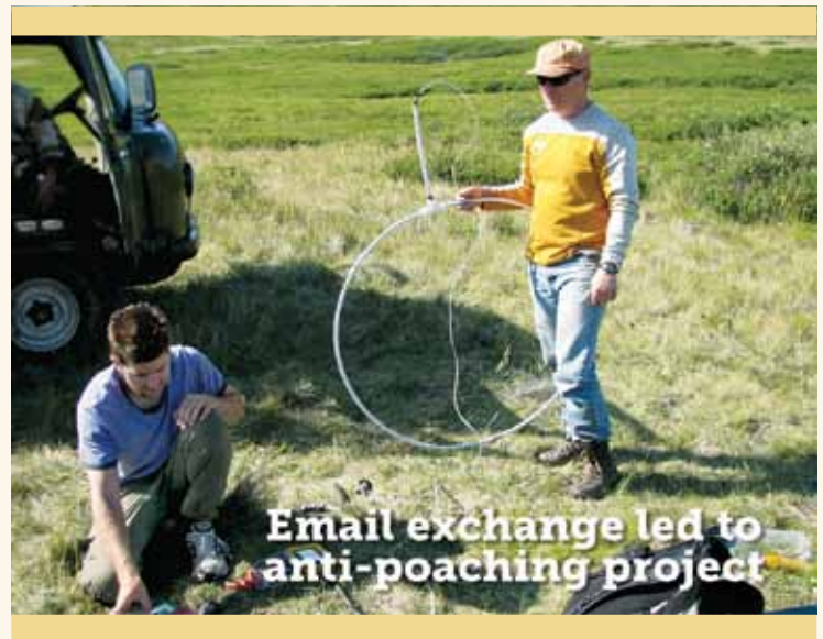
Greg Carney, left, conducts tests on a metal sensor before installation. Sean Burnett holds a weather-proofed sensor coil that will be buried in a roadway.
